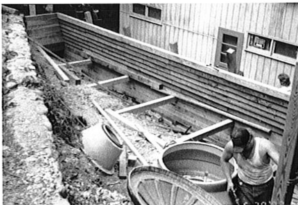
Example of an alternative system being put in on a steep slope.
